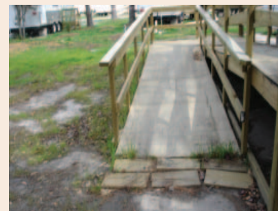
A temporary ramp that needs to be replaced.
